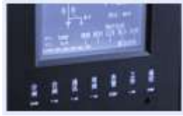
Power System Automation
