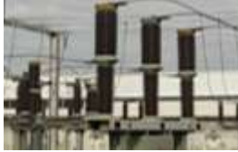
High Voltage System
